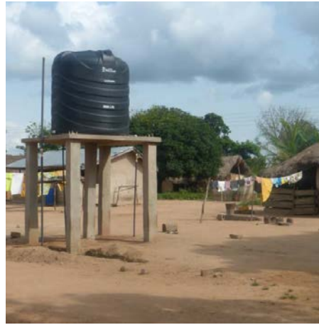
AFTER: A mechanized borehole and overhead tank provides potable water to the community.
